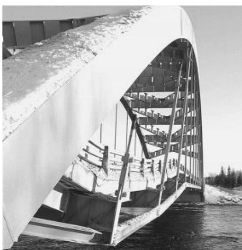
Figura 1. Colapso parcial da ponte Sergeant Aubrey Cosens.
